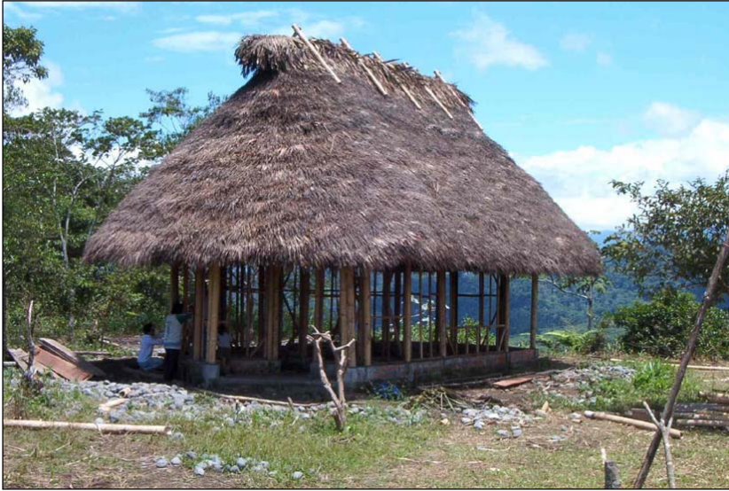
Fig.4: Native Bamboo house rebuilt in the Amazon of Ecuador, by Arq. Ladisich in 2002.
